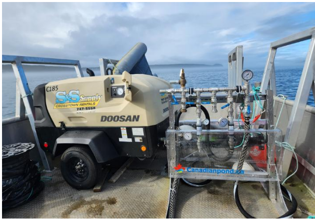
FIGURE 8: COMPRESSOR (LEFT) AND MANIFOLD (RIGHT)
